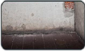
The floor in this house has sunk causing it to separate from the wall.
